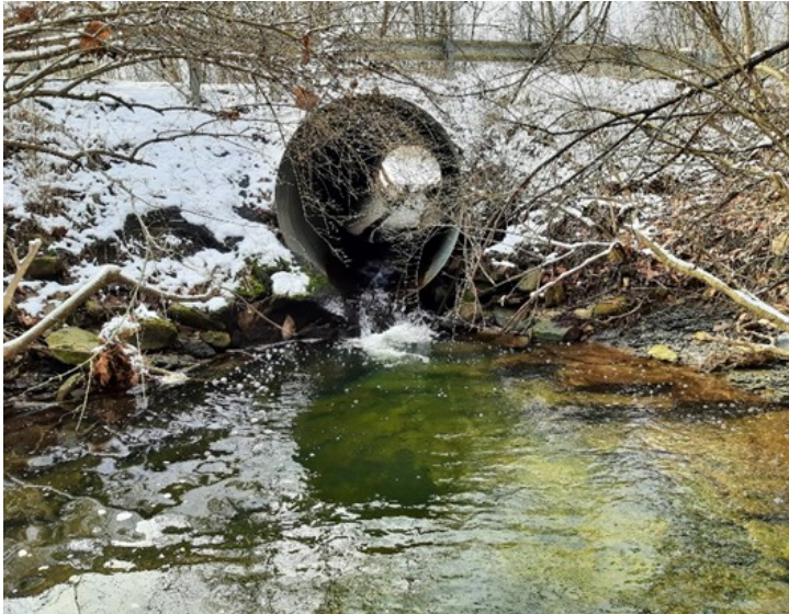
Outlet and "scour" hole at downstream side of the existing culvert pipe under Phillip's School Road.
