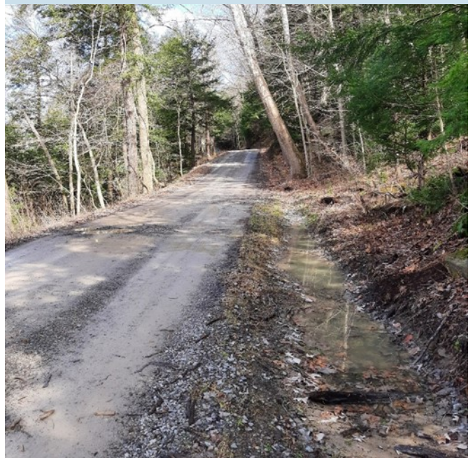
A section of Muddy Creek Road where water is trapped in the road causing wet ditches and potholes.
